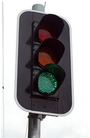
LED traffic lights use 80 - 90% less electricity and have a longer life than regular traffic signals that use incandescent bulbs.
