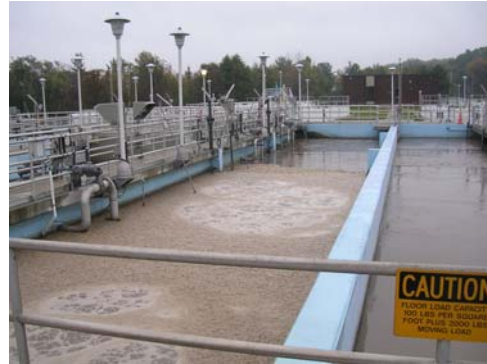
Aeration basins at the Little Patuxent Water Reclamation Plant are a source of nitrous oxide (N 2 O), a potent GHG.
