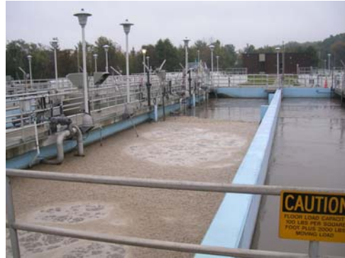
Aeration basins at the Little Patuxent Water Reclamation Plant are a source of nitrous oxide (N 2 O), a potent GHG.
